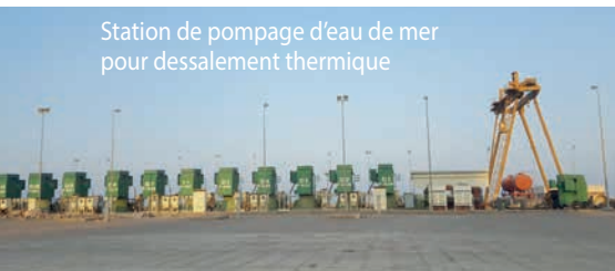
Station de pompage Eau potable
