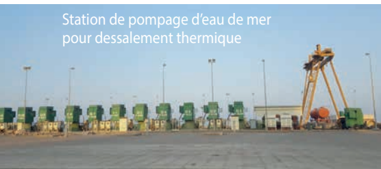
Station de pompage Eau potable
