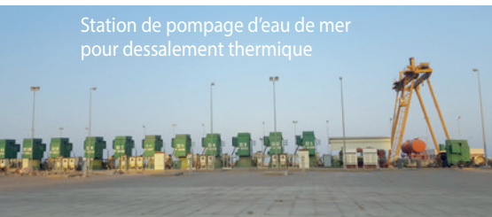
Station de pompage Eau potable
